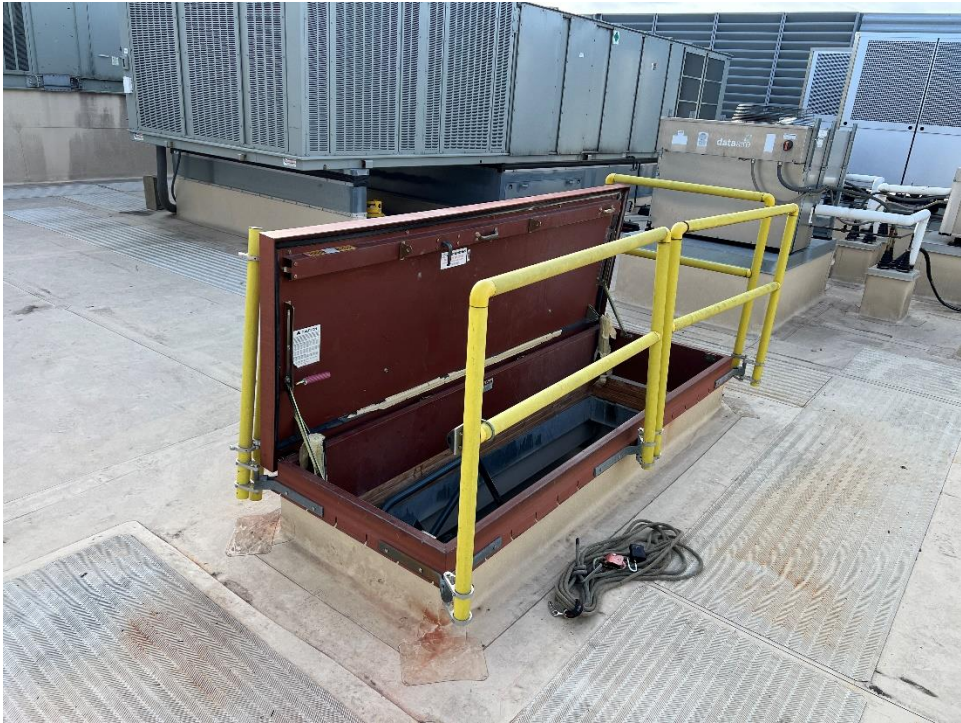
Photo 6: Non-compliant roof hatch access.
