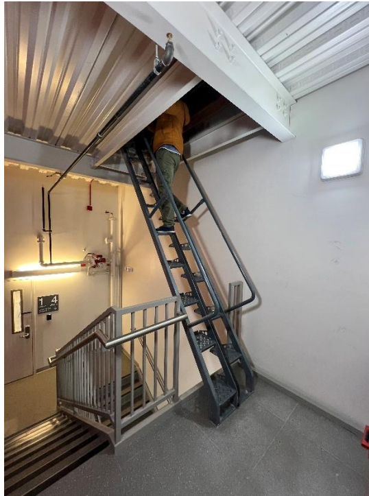
Photo 7: No fall protection system drawing present by the roof/system access point.
