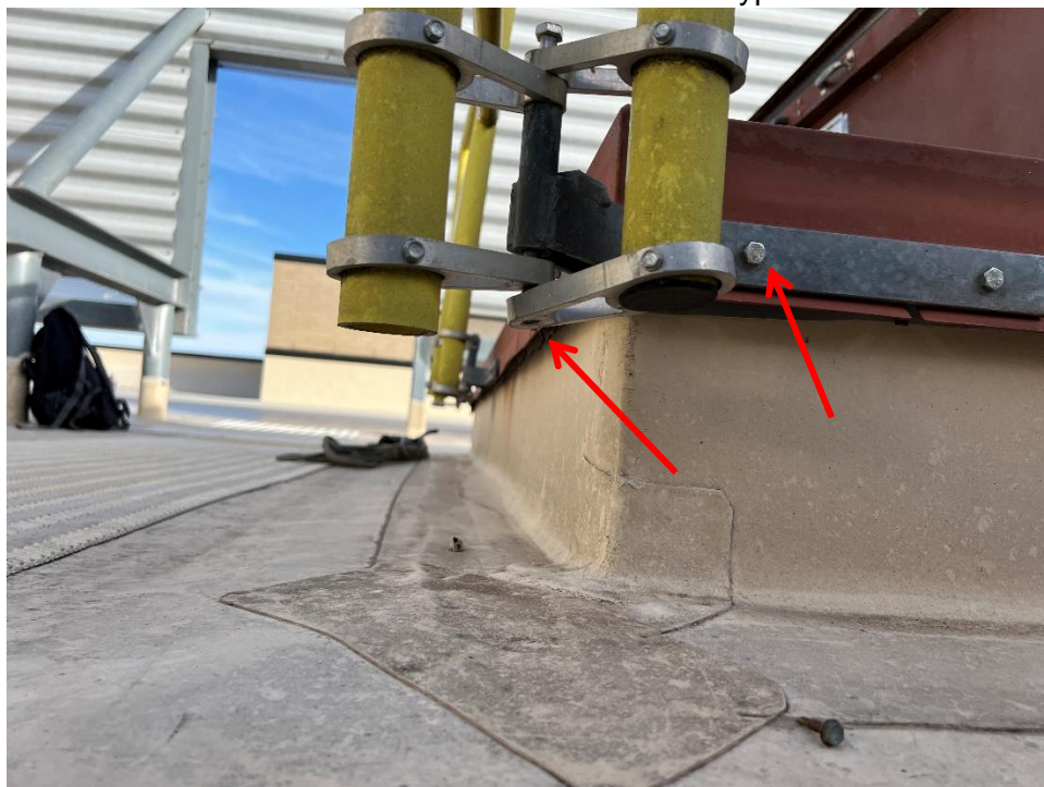
Photo 2: Missing locking nut at the corner connection. Typical. No washer at the bolted connection. Typical.
