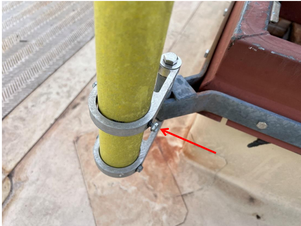
Photo 3: Loose self-tapping screw. Typical.
