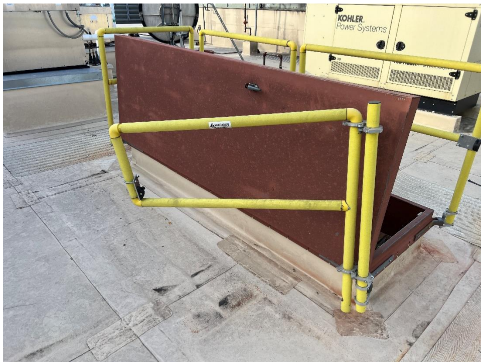
Photo 4: Self-closing swing gate does not close on own.
