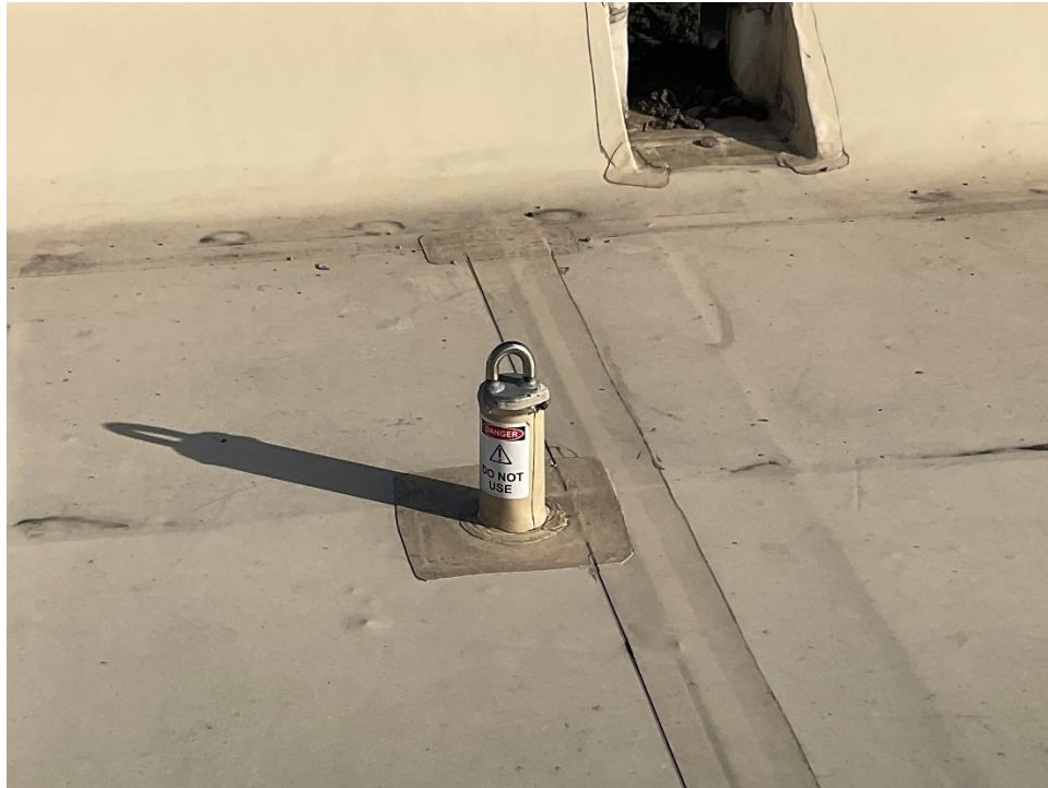
Photo 1: Uncertified single point fall protection anchor tagged with a DANGER – DO NOT USE sticker. Typical.
